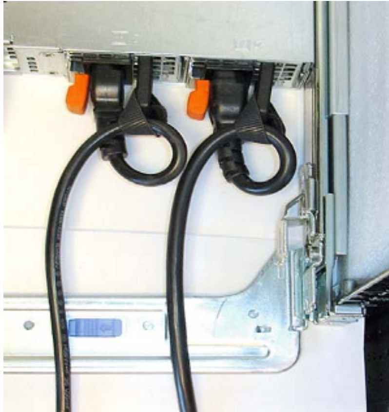
Figure 23: Proper PSU Cabling
