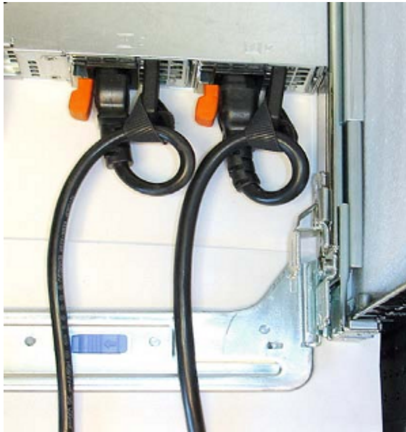
Figure 23: Proper PSU Cabling
