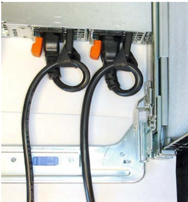
Figure 23: Proper PSU Cabling
