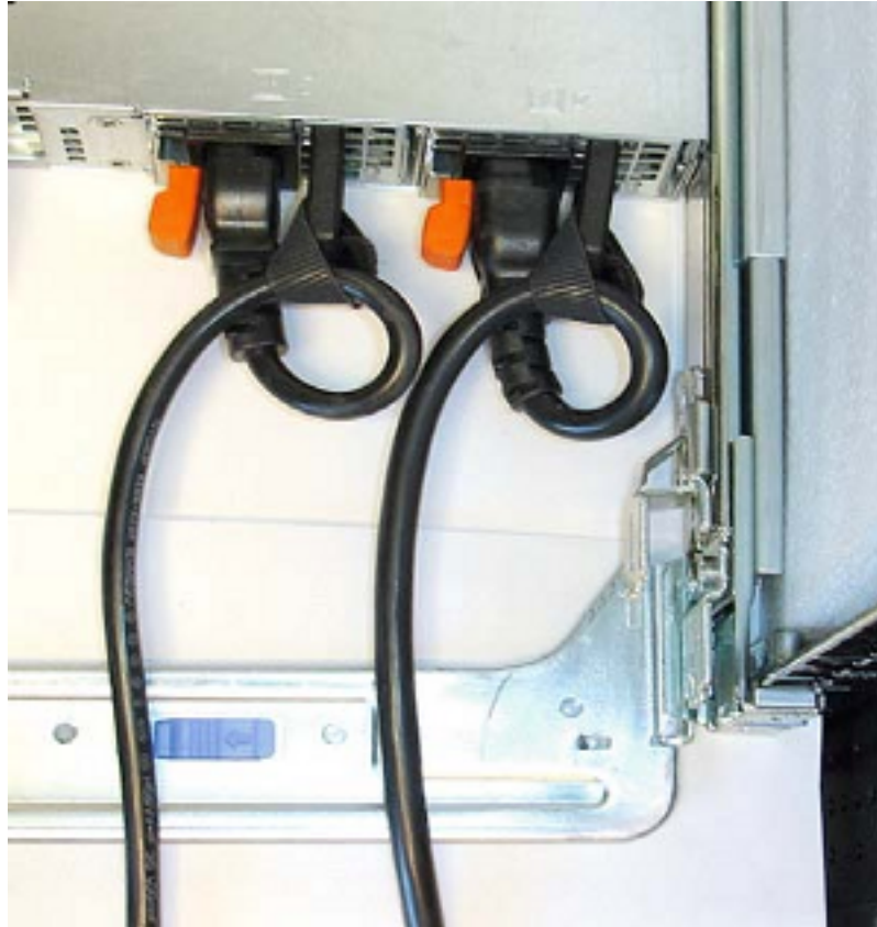
Figure 12: Proper PSU Cabling
