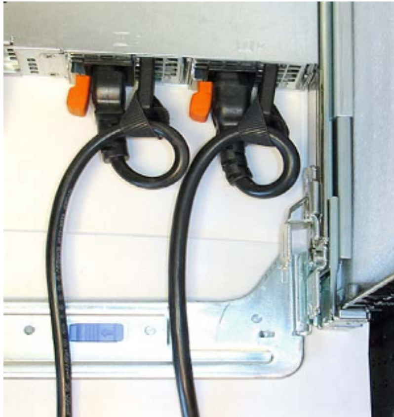
Figure 12: Proper PSU Cabling
