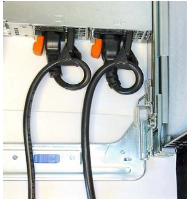
Figure 10. Proper PSU Cabling
